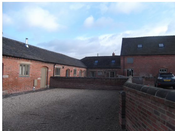
Picture B.5 An example of localised repointing
