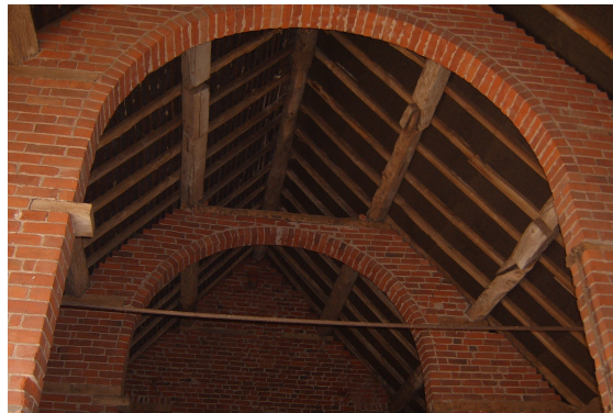
Picture B.10 An example of an open plan interior which allows the roof structure to remain exposed
