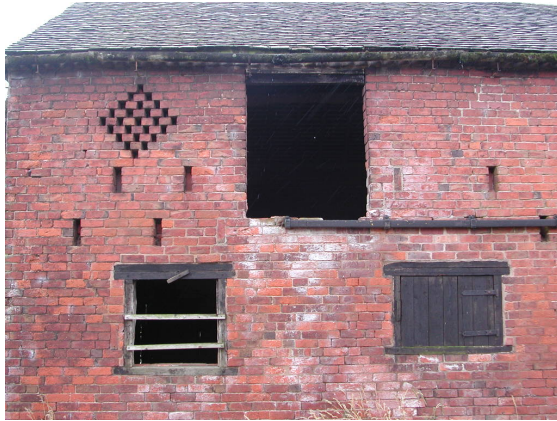
Picture B.11 Picture shows important features which should be identified and retained as part of any refurbishment
