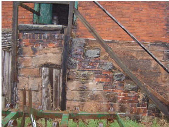
Picture B.12 External stairs are an example of a feature which should be identified and retained as part of any refurbishment
